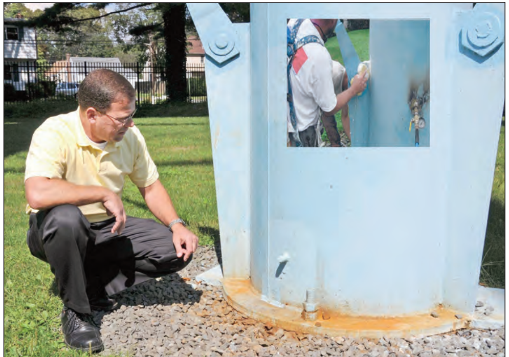
Superintendent Stan Carey inspects recent work performed on the District's elevated storage tank at May Place. Through a proactive infrastructure maintenance program water was discovered in one of the support legs and was addressed immediately. The District's tank engineer using a state of the art underwater remote operation vehicle (ROV) confirmed the structural integrity of the tank had not been compromised.
